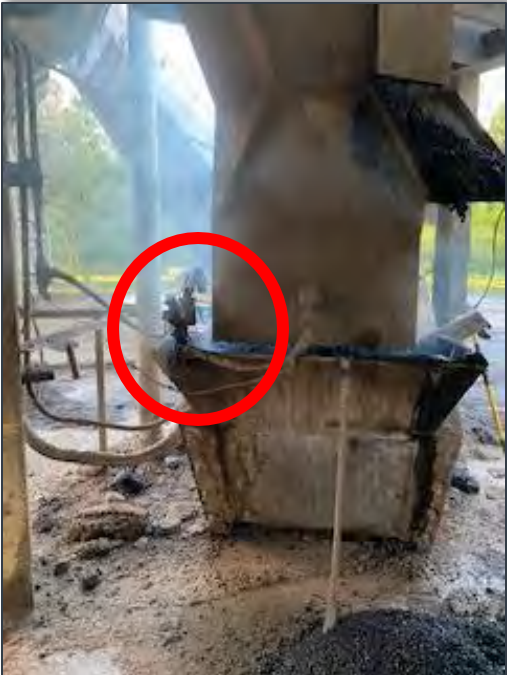
One particulate analyzer placed over the chute
